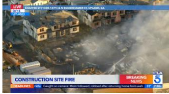
Construction Fire Site in Upland
