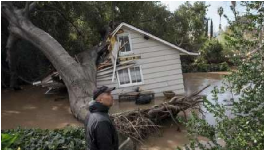
San Jose resident Rob Souza surveys damage to a guest house on William Street near Coyote Creek on Feb. 2.
