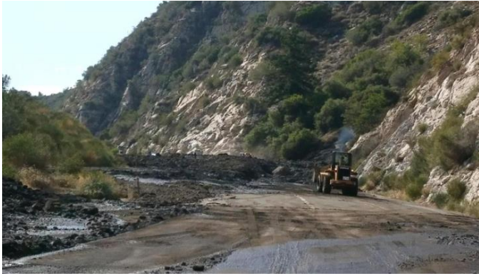
Dozers work to clear Highway 38 near the Valley Fire on July 7 following a mudslide. Photo courtesy of IC
