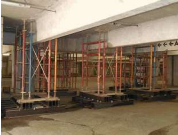
The parking garage at Lake Arrowhead Village remains closed while undergoing seismic retrofitting. (Photo by Rhea-Frances Tetley)
