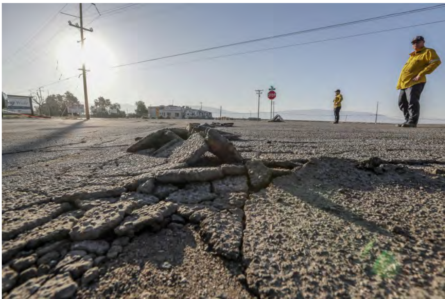
Buckled asphalt in a parking lot in Argus, Calif., after the Ridgecrest earthquakes in July. (Robert Gauthier / Los Angeles Times)
