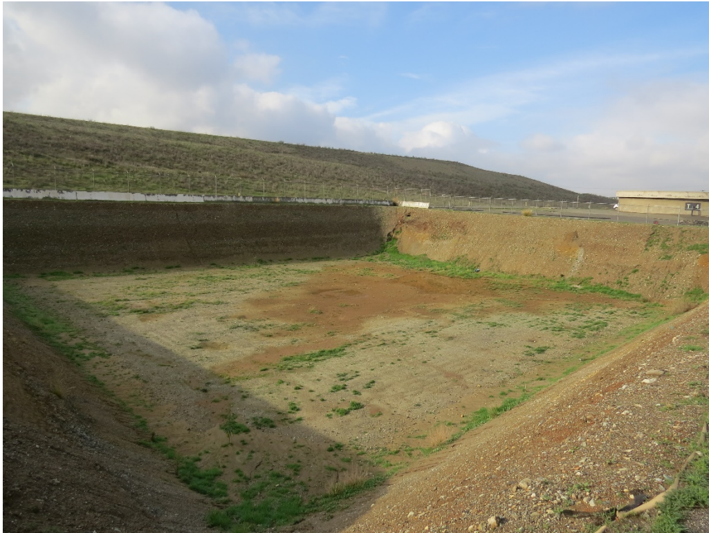
Photograph 9: Looking at the excavated basin near the southeast corner of the project site.
