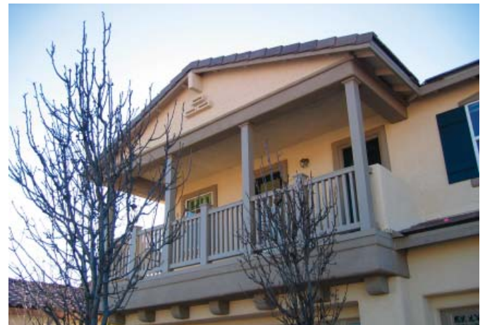
Stucco or plaster exterior, sometimes with wood siding on the second story
