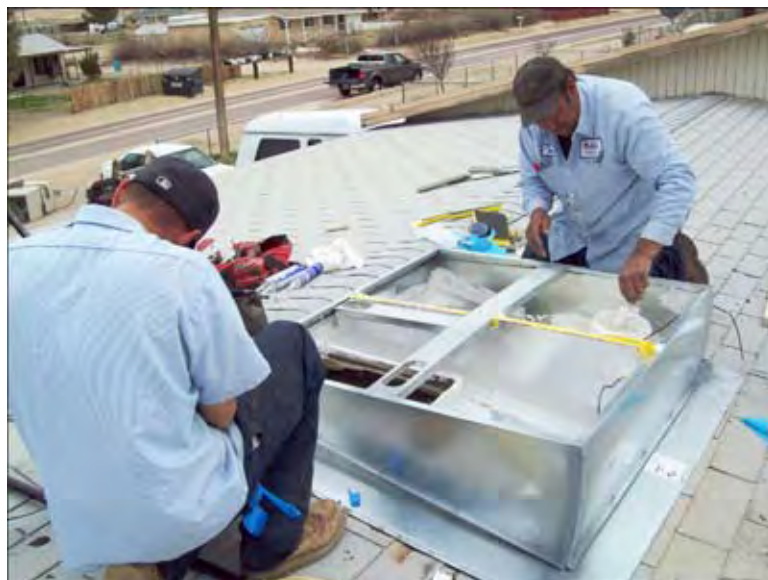
CAPSBC Weatherization Crew Technicians seal off the base of an air conditioning/heating unit to prevent air from escaping to the outside of the home.
