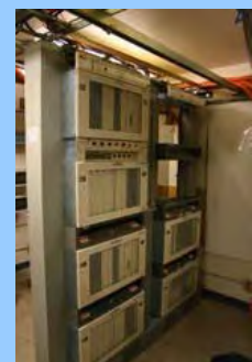
Digital access cross-connect system located in the High Desert, used to transmit public safety radio signals to outlying areas
