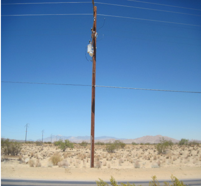
Photograph 9: Looking west at the generation line extension along Sunfair Road just north of Pipeline Road.
