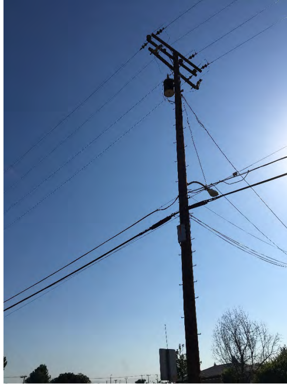
Photo 13 – One of the pole-mounted transformers on the Property.
