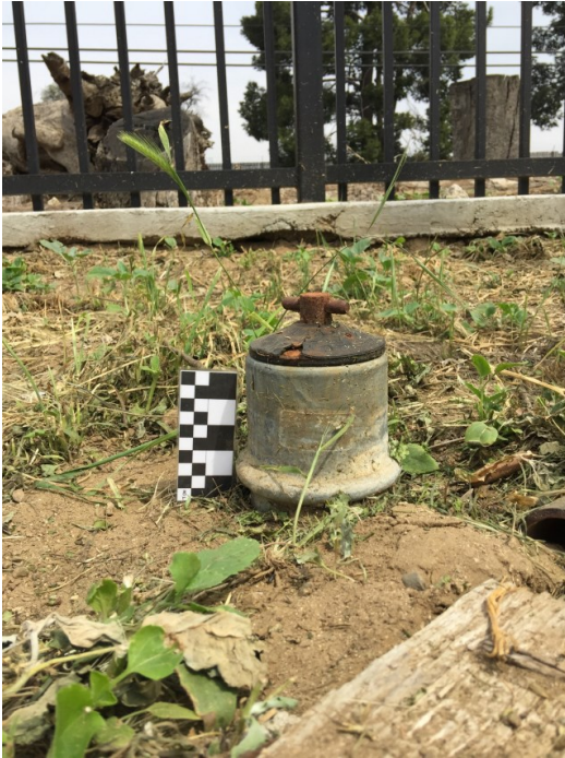
Photograph 2: Close-up of the Irrigation Valve.
