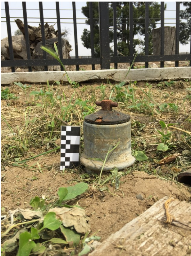
Photograph 10. Close-up of the Irrigation Valve from SCA-1.
