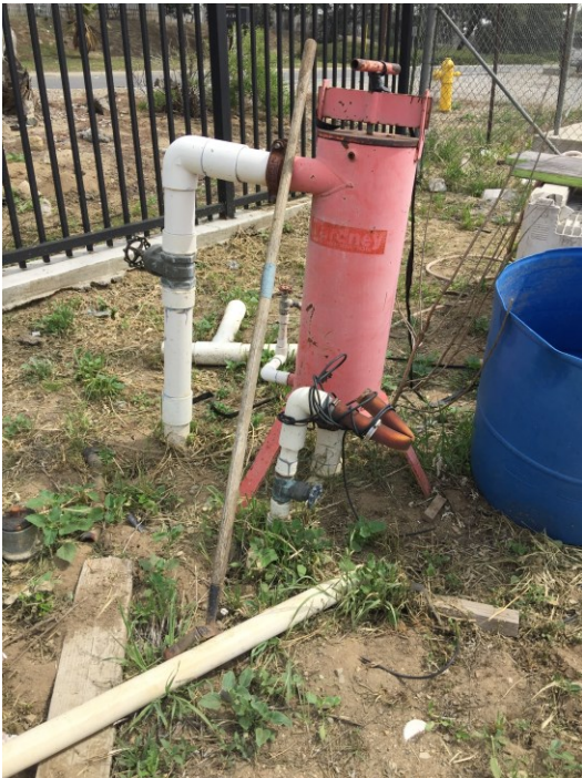
Photograph 3: Close-up of the Well Pump.
