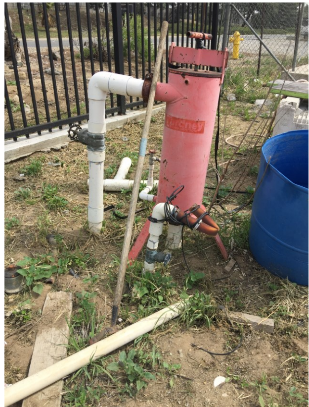
Photograph 11. Close-up of the Well Pump from SCA-1.
