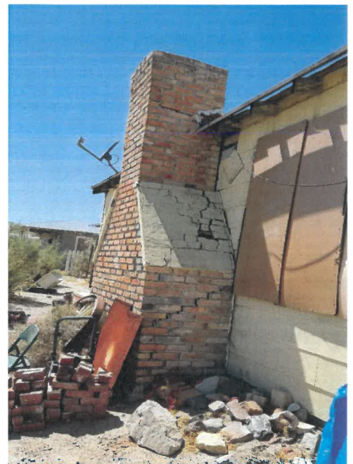
Figure 2: Chimney damaged in Trona Earthquake
