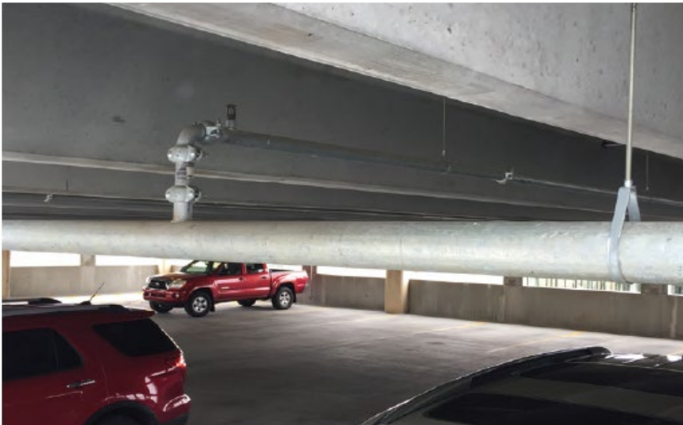
Sprinklered open parking garage.
