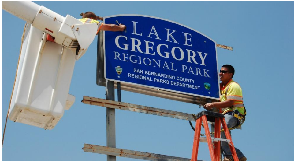
A crew from Hi-Way Safety installs the new Lake Gregory Regional Park sign along Highway 18 in San Bernardino
